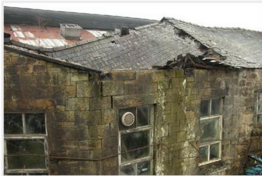
Photo 7: Poor condition of roof to Pattern Maker's Workshop.
